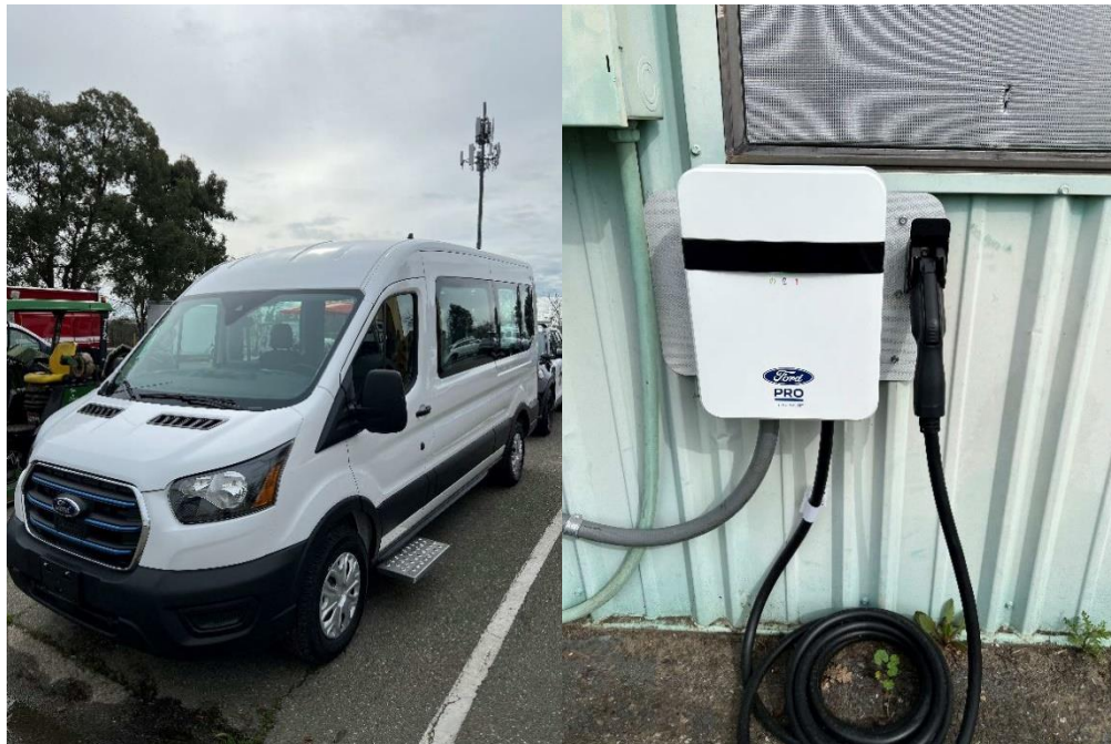
Fig 1. and Fig 2. The City of Davis’s new electric van and charger, March 2024
