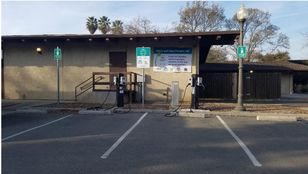
Winters Community Center Operational Chargers with permanent aluminum sign and temporary banner
