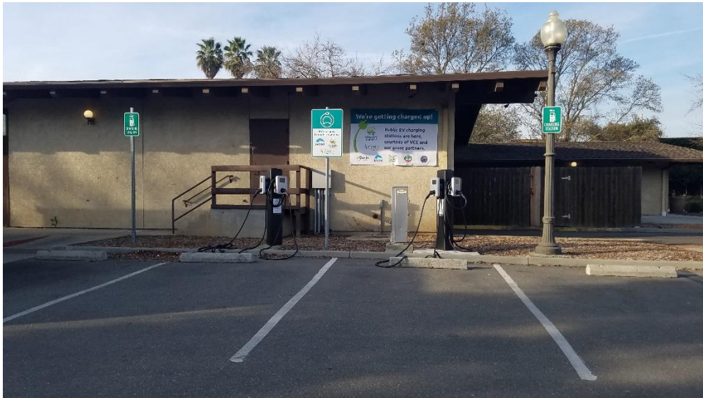
Winters Community Center Operational Chargers
